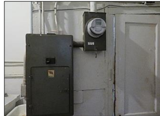
ELECTRICAL SYSTEM; Overhead service drop inlet wires- 100 Amperes- breaker type
