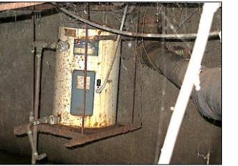
WATER TANK HEATER; Electric type; located on crawl space.
