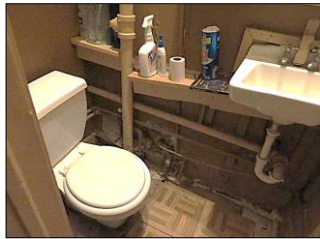
1/2 BATHROOM; Wooden doors- vinyl floor tiles- wooden sash windows- vent fan- light fixtures.
