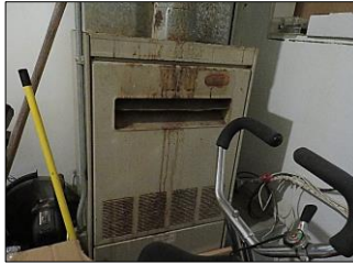
HEATING SYSTEM; LENNOX brand- natural gas system- approximately 20 years older.
