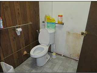
1/2 BATHROOM; Wooden doors- vinyl floor tiles- vent fan- light fixtures- wooden vanities- sink and fixtures
