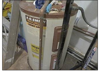
WATER TANK HEATER; A/O SMITH brand- natural gas type- 30 U S gallons 1989.
