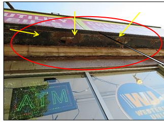
EXPOSED HANGING LIGHTS ON WIRES
