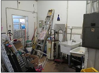
UTILITY ROOM; Wooden doors- wood floors- light fixtures- furnace- water tank heater- electrical panel box- furnace- laundry sink.
