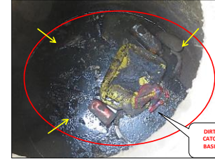
MISSING DOWN SPOUT EXTENSION
