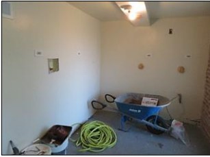
Sample pictures of LAUNDRY ROOM: Steel doors - painted concrete floors - light fixtures - drywalls.
