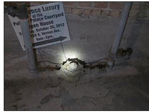
MAIN WATER METERS/ CUT OFF VALVE : Located on basement area
