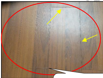
SAMPLE PICTURES OF DAMAGED AND LOOSE KITCHEN FLOOR COVERINGS
