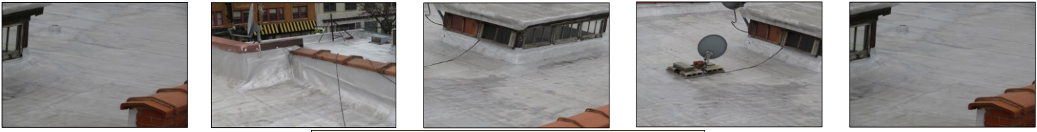
Sample pictures of ROOFING SYSTEMS: Flat rubber roof, roof tiles - steel gutters and down spouts
