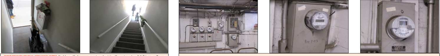
FRONT COMMON STAIRS & LOBBY (13121 ENTRY): Steel doors with glass panes - carpet wooden stairs with carpet coverings - light fixtures - mailboxes - drywalls - radiator heater. ELECTRICAL SYSTEMS: Overhead service drop inlet wires - STABLOCK/FEDERAL PACIFIC/PUSHMATIC BREAKERS - 150 Amperes, step down to 100 amperes per unit - located on basement areas and sub panel on each unit.
