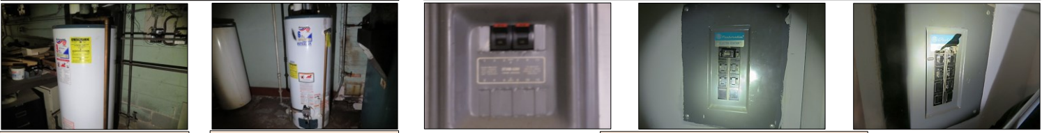
WATER TANK HEATER: Conventional - gas type - RICHMOND Brand - Model # 7K50 SERIAL # RMNG080218054 - CAPACITY - 50 U S GALLONS YEAR MANUFACTURED - 2000 - Located on basement area. WATER TANK HEATER: Conventional - gas type - RICHMOND Brand - Model # 6G50 SERIAL # RMALN267517655 - CAPACITY - 50 U S GALLONS YEAR MANUFACTURED - 12/2007 - Located on basement area. Sample pictures of Electrical PUSHMATIC panel box on each unit
