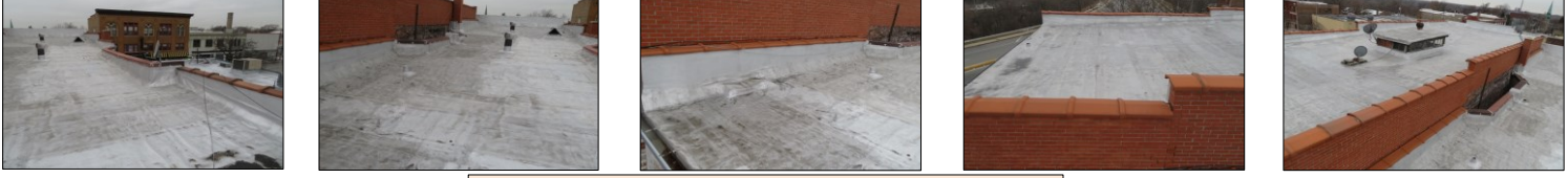
Sample pictures of ROOFING SYSTEMS: Flat rubber roof, roof tiles - steel gutters and down spouts
