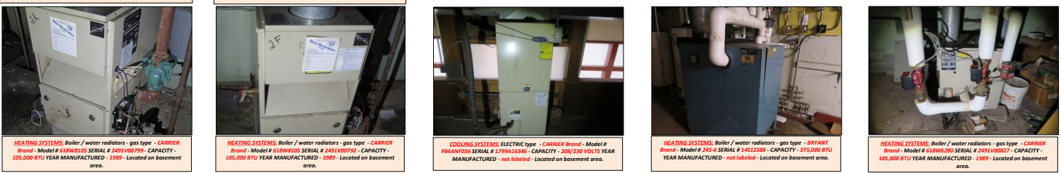
HEATING SYSTEMS: Boiler / water radiators - gas type - CARRIER Brand - Model # 618W6105 SERIAL # 2491V00759 - CAPACITY - 105,000 BTU YEAR MANUFACTURED - 1989 - Located on basement area. HEATING SYSTEMS: Boiler / water radiators - gas type - CARRIER Brand - Model # 618W6105 SERIAL # 2491V00752 - CAPACITY - 105,000 BTU YEAR MANUFACTURED - 1989 - Located on basement area. COOLING SYSTEMS: ELECTRIC type - CARRIER Brand - Model # F84ANF36 SERIAL # 1799A16346 - CAPACITY - 208/230 VOLTS YEAR MANUFACTURED - not labeled - Located on basement area. HEATING SYSTEMS: Boiler / water radiators - gas type - BRYANT Brand - Model # 245-S SERIAL # 14512580 - CAPACITY - 375,000 BTU YEAR MANUFACTURED - not labeled - Located on basement area. HEATING SYSTEMS: Boiler / water radiators - gas type - CARRIER Brand - Model # 618W6290 SERIAL # 2491V00827 - CAPACITY - 105,000 BTU YEAR MANUFACTURED - 1989 - Located on basement area.
